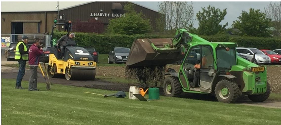
A new patio area has been laid for our picnic benches and even the driveway has had a revamp
